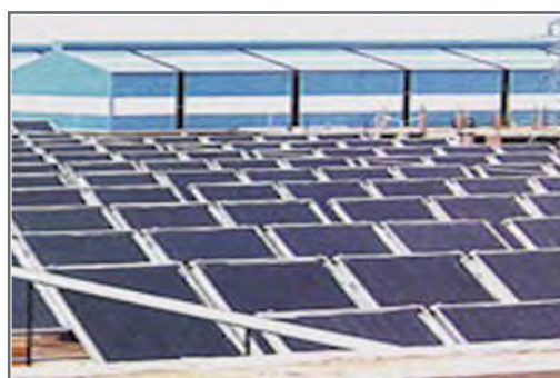
Fig 3.15: Solar Panels to trap solar energy
